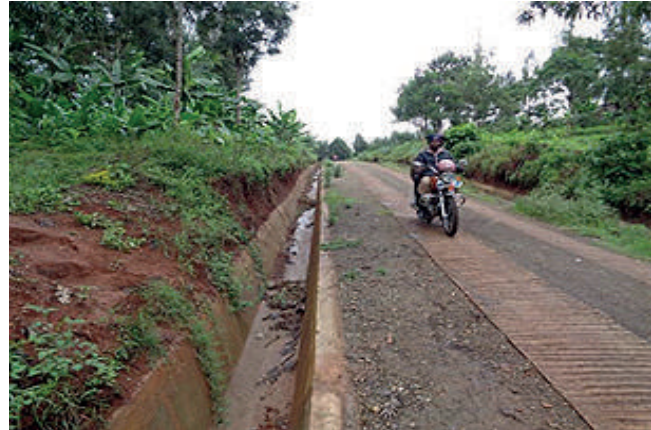
Figure 10-13: Inappropriate choice of roadside drain (Leaves no room for recovery if a vehicle runs off the road)
