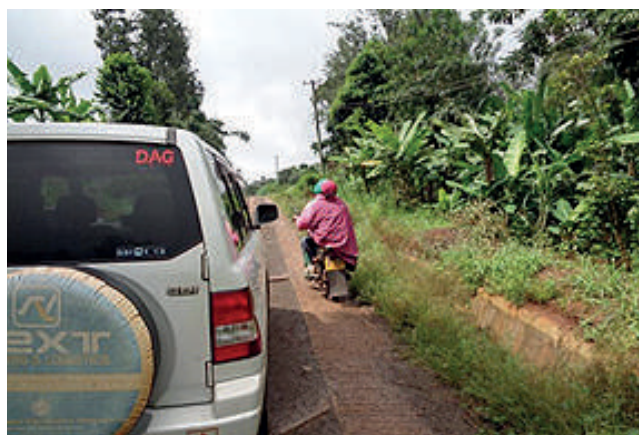
Figure 10-5: Problems encountered on concrete strip road
